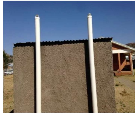
Figure 2. Back view of VIPs at a large hospital facility in Lesotho (note the white vent pipe and fly screen (capping pipe) with very large holes).
